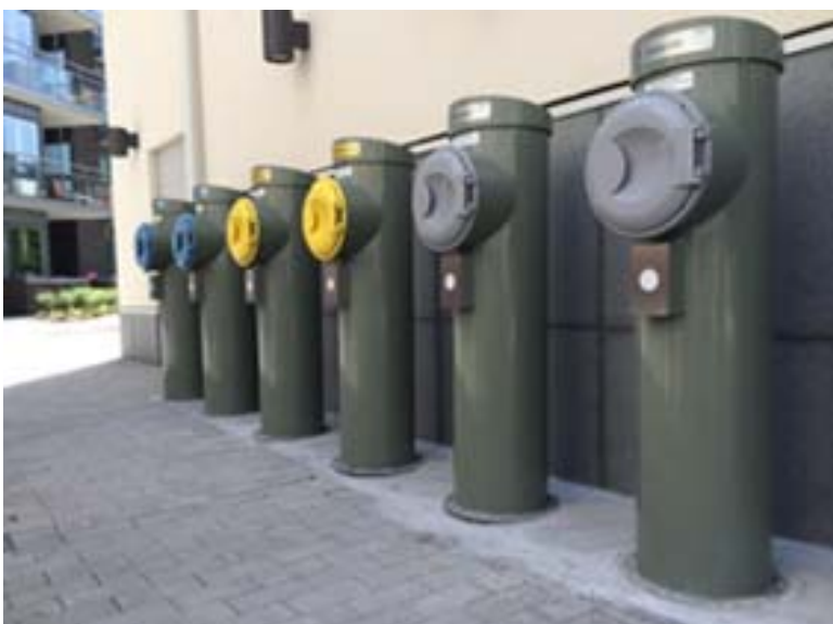
Stockholm Royal Seaport advanced recycling center installed in a residential complex, Stockholm, Sweden
